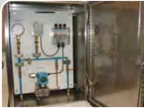
Pressure Manifold Cabinet Water Industry
